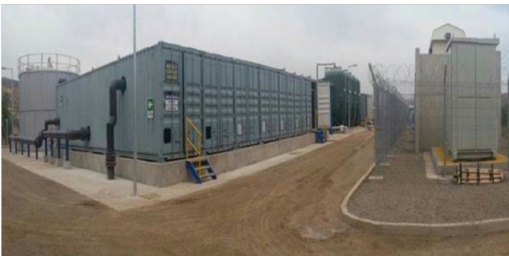
View of the nanofiltration containers at the plant.
