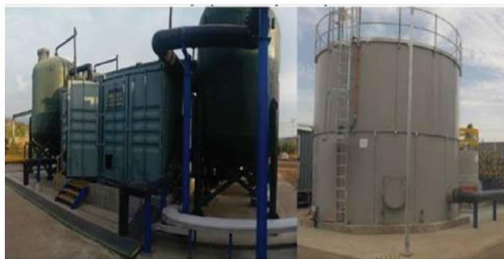
Sand filters and runoff tank.
